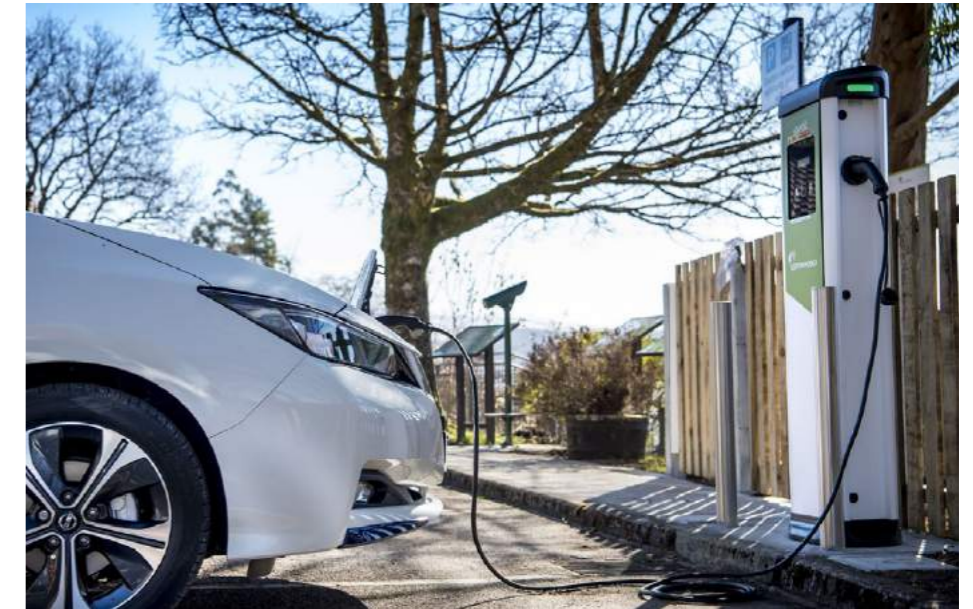
Fig. 22 - Electric vehicle charging point.
