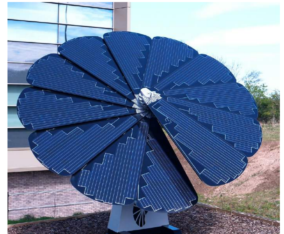
Fig. 24 - Existing solar panels installed on SAEZ site.
